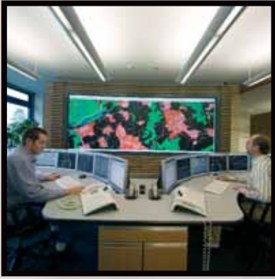
The ZNL Esslingen is equipped with 4 display walls each consisting of 4x2 OVERVIEW mDG50-DL projection modules and a TRANSFORM A controller
