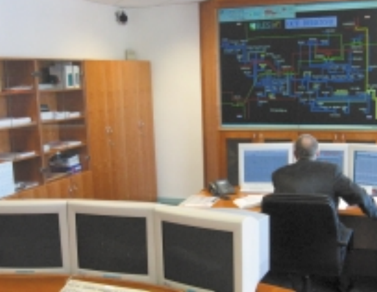
ELES' training center includes an OVERVIEW MP50 display wall with 2x2 projection modules for realistic and efficient operator training
