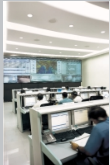
Security Control Room (67" modules in a 5x2 configuration).
