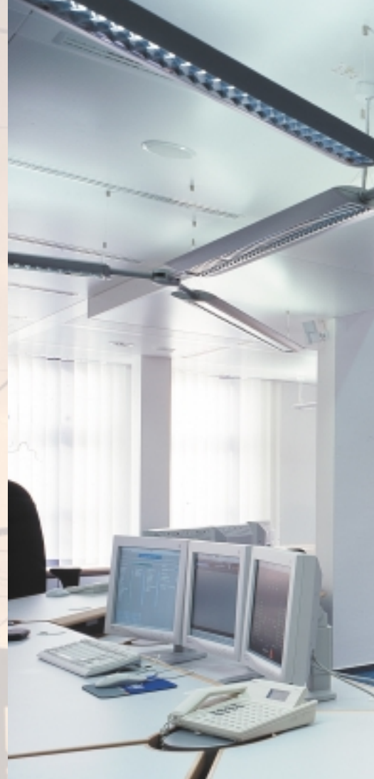
In the control center at Stadtwerke Düsseldorf AG, the energy network management area is equipped with a 4x3 OverView mP50 rear-projection display wall and the technical service center with a 3x3 OverView mP50 rear-projection display wall, both controlled by Barco's Eos graphics controllers
